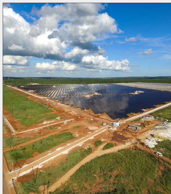
An areial view of the IDC's first greenfield project, the 54 MWp solar photovoltaic plant in Lusaka.
